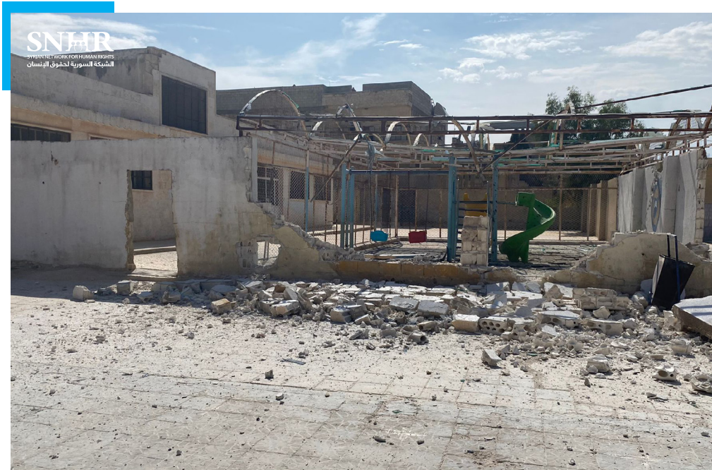
👁 Destruction and damage at the Hussein Haj Abboud School for Elementary Education in Sarmin city in eastern rural Idlib governorate following a regime rocket attack - October 5, 2023 © SNHR
