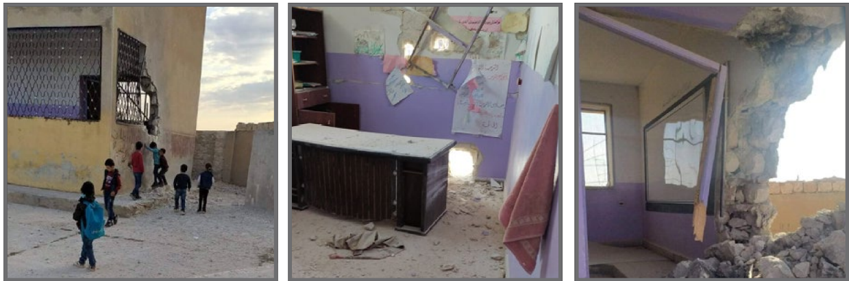
Pictures showing the damage caused to Ma'ar Ballit School by bombing by Syrian regime artillery forces - November 4, 2022
