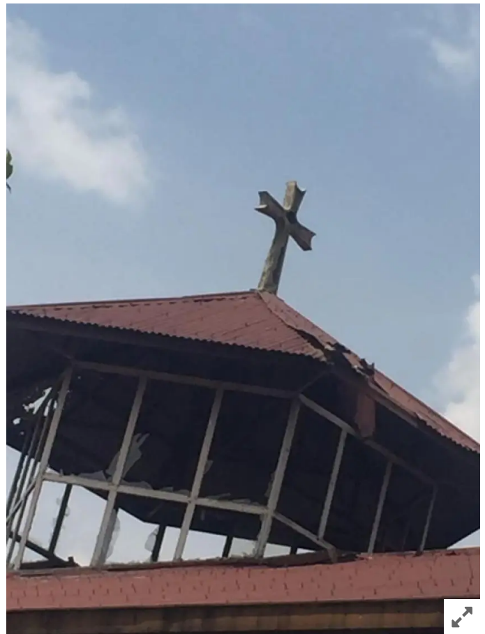
A church in Kitchanga, Masisi territory, damaged during attacks by the M23 in January 2023. © 2023 Private
