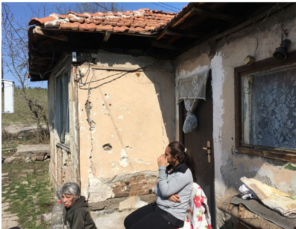
The cracked house belonging to Maria in the neighbourhood of Rudnichar in Pernik, Bulgaria. Photo supplied by Vesselina Foteva.
