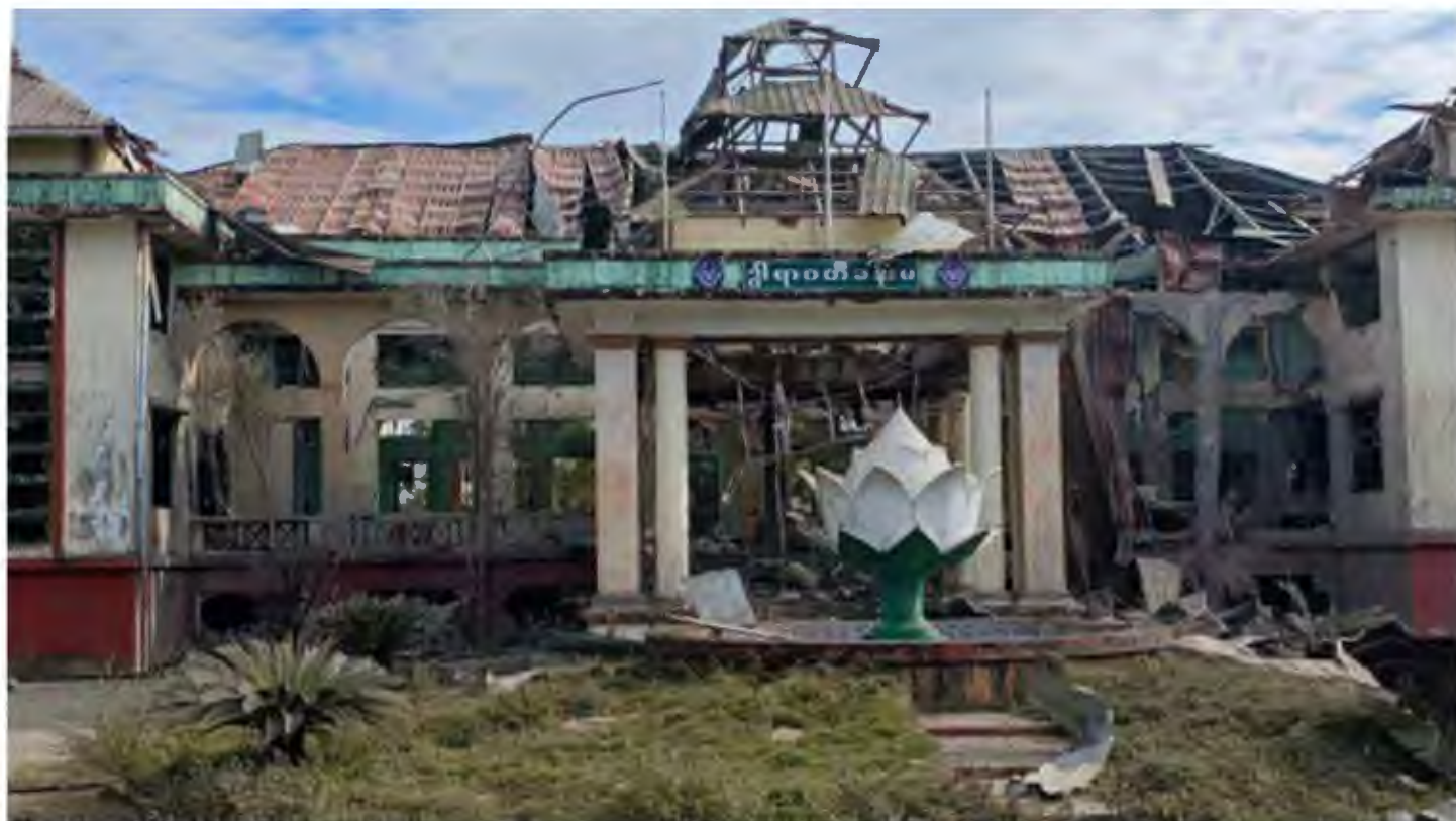
Buildings in Rakhine state's Thandwe township destroyed by junta bombs on Sept. 26, 2024. (Arakan Princess Media-Telegram)
