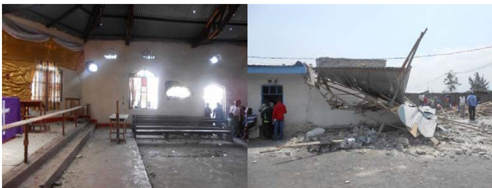
Left: Anglican church. Right: Damaged school.
