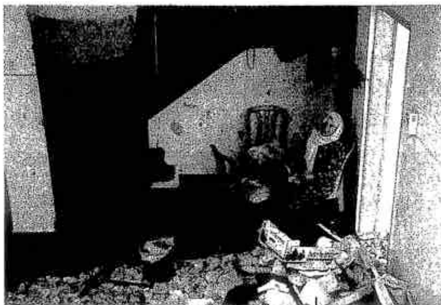
Woman sitting in the remains of her house in al-'Ayn refugee camp in Nablus. Her house was irreparably damaged when the army destroyed her neighbour's house in a punitive demolition in October 2002. © Amnesty International
