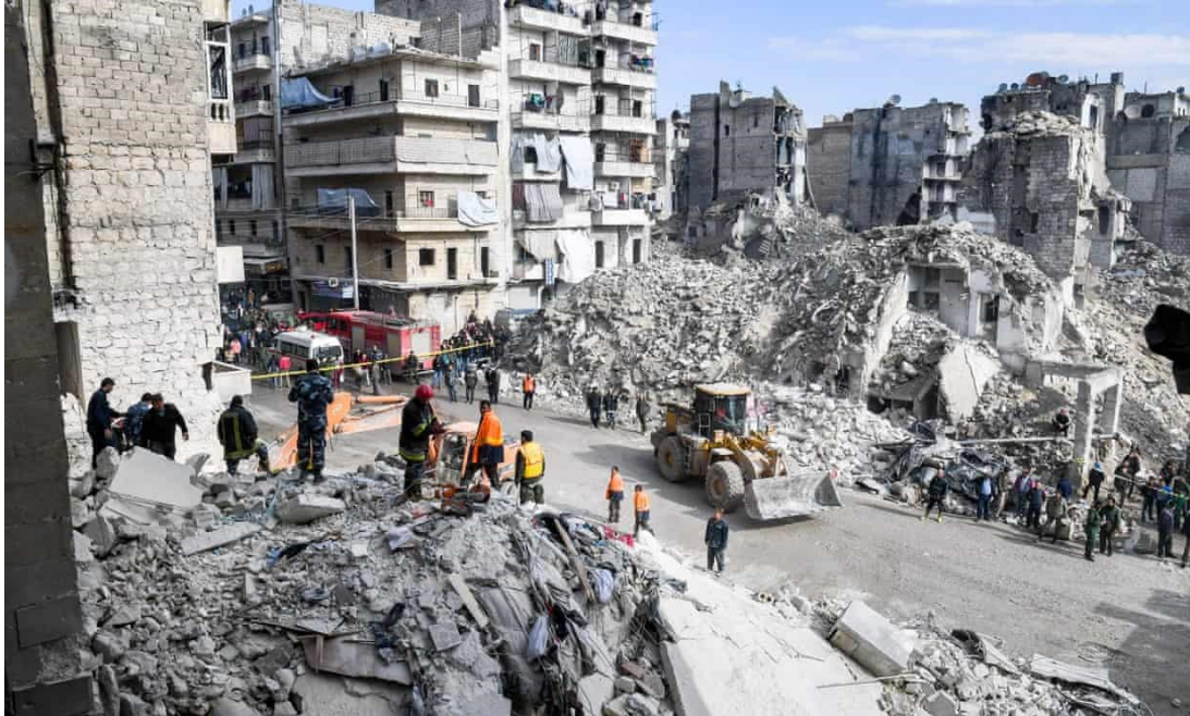
Syrian civil defence workers search the rubble of the collapsed building in Aleppo
