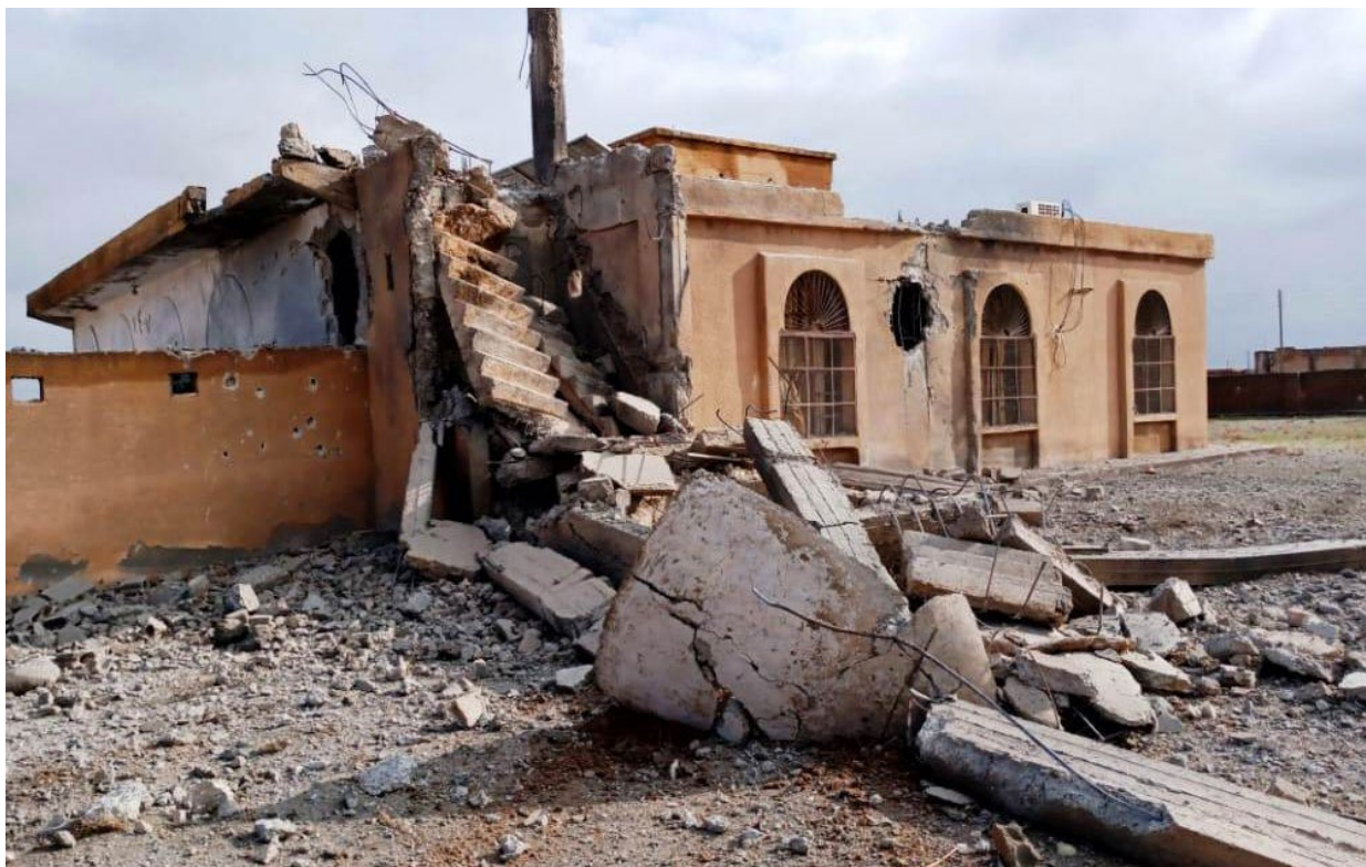
Destruction in the aftermath of a ground-based attack originating from an SNA-held area on Abu Bakr al-Siddeeq Mosque in al-Trowaziya village - December 1, 2022
