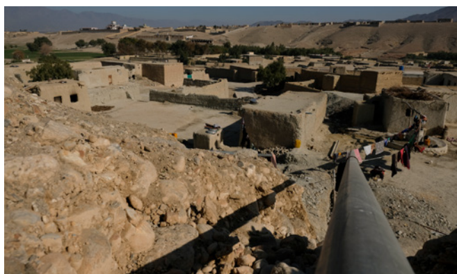
The 2,600-metre water pipe system runs down from the main water reservoir (which holds 60,000 litres of water) bringing vital water to a small village in Behsud District of Jalalabad. ©UNHCR 2017/S. Rich
