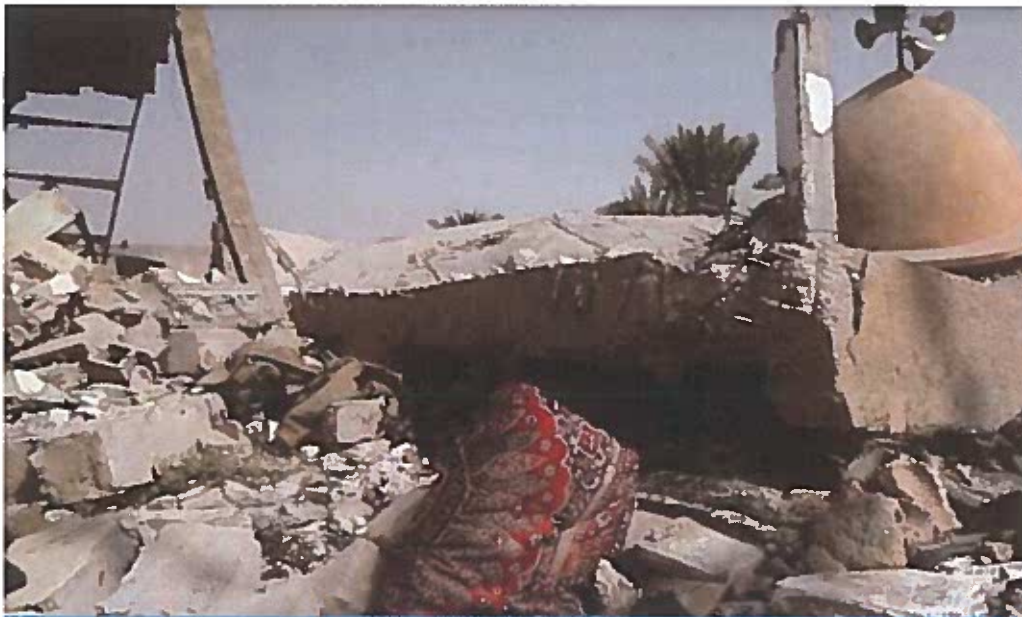
Destruction to the Ammar bin Yasser, formerly al Mustafa Mosque, in the aftermath of an attack by international coalition forces on al Susa town in Deir Ez-Zour – October 19, 2018
