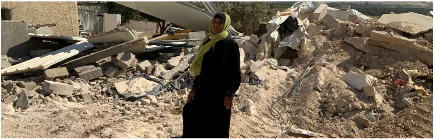
A Palestinian woman was displaced after Israeli forces demolished her house for lack of an Israeli-issued building permit, which is almost impossible to obtain, Jericho. Photo: OCHA
