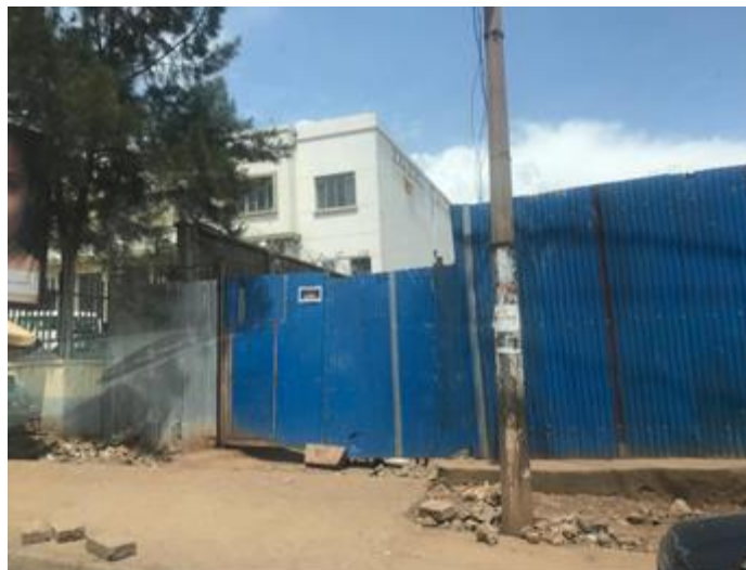
Congo Gold Raffinerie (CGR) construction site, Bukavu, South Kivu (photograph taken by the Group in March 2020)
