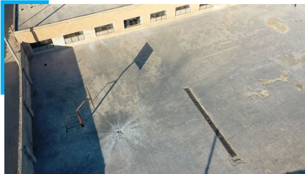
↑ 👁 Damage caused by a ground attack by Syrian regime forces on the Shuhada Afis School in Afis village in Idlib - December 2, 2023
