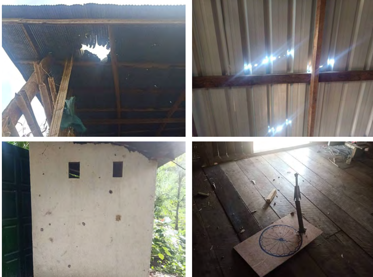
These photos were taken on June 3 rd 2021, in U--- village, Kaw T'Ree Township, Dooplaya District. They show the damage to villagers' houses that was caused by the firing of mortars and bullets. [Photos: local villager]
