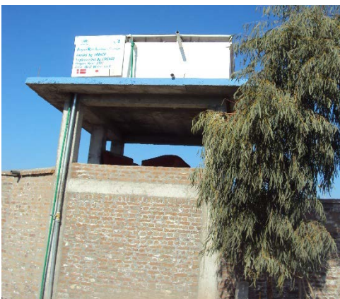
View of the water reservoir constructed by UNHCR in SMNT@ UNHCR/ Eamal
