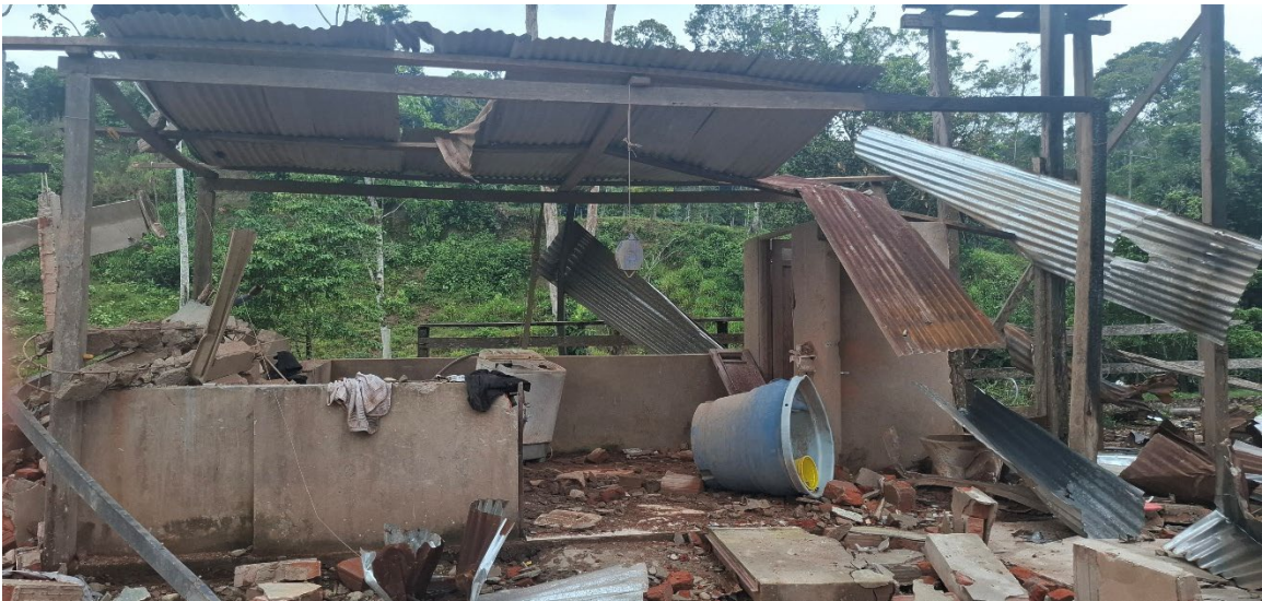
Two photographs of the damage caused to the property burned on March 3 and bombed on March 6, 2026. © 2026 Alliance for Human Rights
