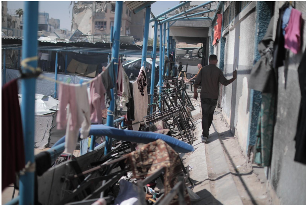
Forcibly displaced people continue to seek shelter in a severely damaged UNRWA school-turned-shelter in Gaza city, the Gaza Strip, April 2025. © 2025 UNRWA Photo
