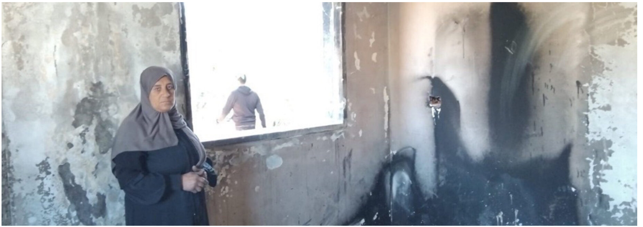
A house belonging to a 65-year-old Palestinian woman and her grandson was severely damaged due to an Israeli settler attack in Jalud village, Nablus. Photo: Partner
