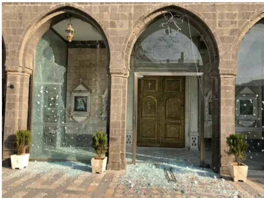
Damage caused by a rocket shell whose source remains unknown on the Church of Lady of al Niaah Cathedral, known as the Zeitoun Church in Bab Sharqi, Damascus – January 9, 2018
