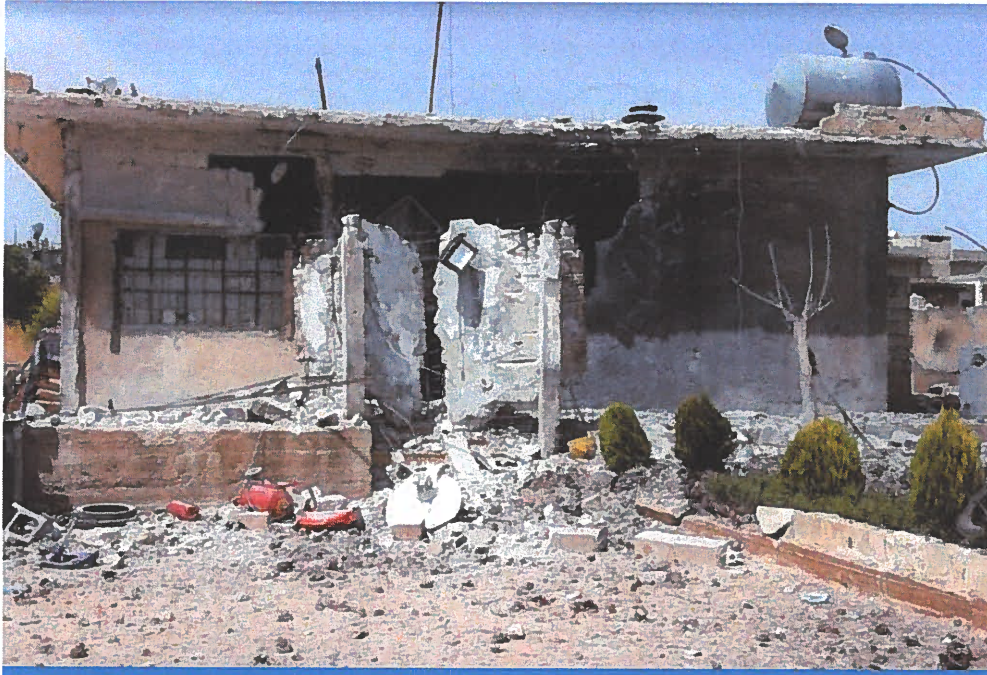
Damage in the '33103' Civil Defense Center in Kafr Nbouda town, Hama, in a Syrian ground attack – May 1, 2019
