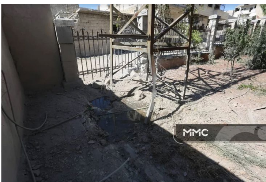
Damage to the Primary Health-Care Center in Ma'aret al Numan city, Idlib inflicted in a ground attack by Syrian Regime forces – October 3, 2019
