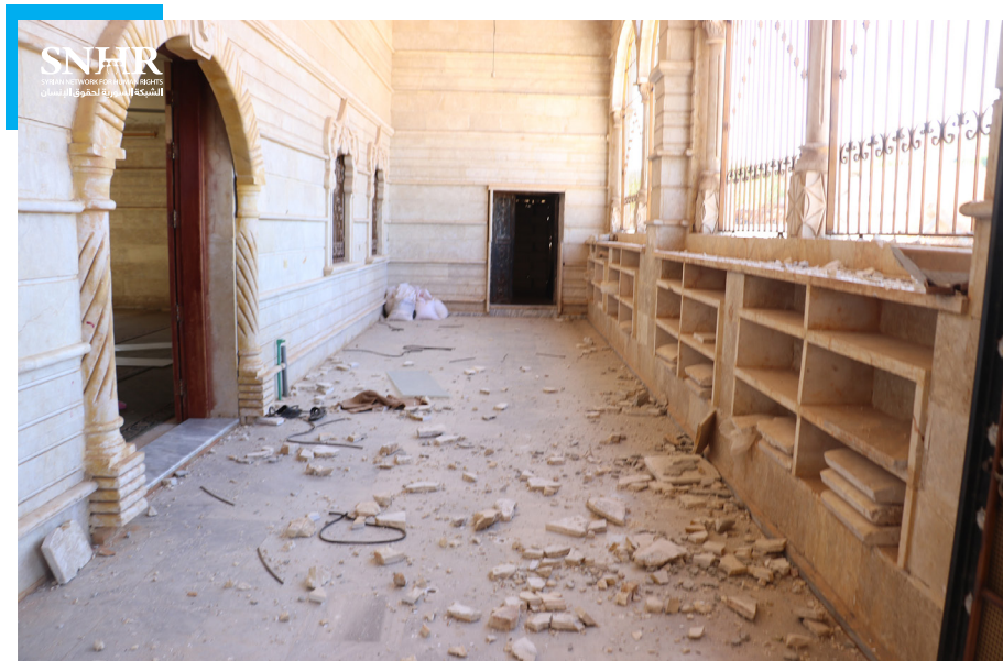
👁 Damage to the Grand Mosque in al-Mozara village in Idlib following a ground regime attack - September 5, 2023 ©SNHR
