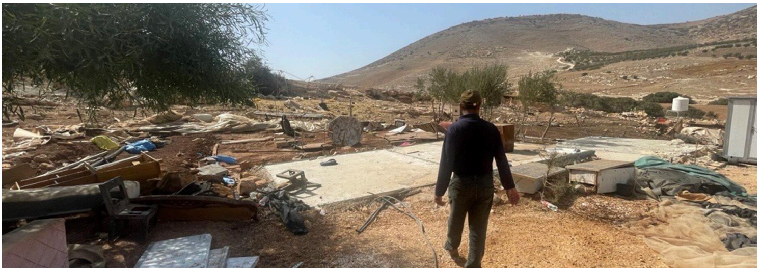
A Palestinian man walks by what remains of the structures that he and his neighbours had to dismantle in Ibziq herding community, in Tubas governorate, following a wave of settler attacks that has forced them to relocate. Photo by OCHA
