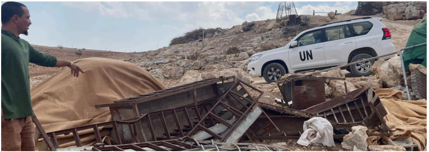
A resident of the Palestinian herding community of Khirbet Tell al Khashaba, in Nablus governorate, showing a UN team what remains of structures that Israeli authorities demolished. Photo by OCHA
