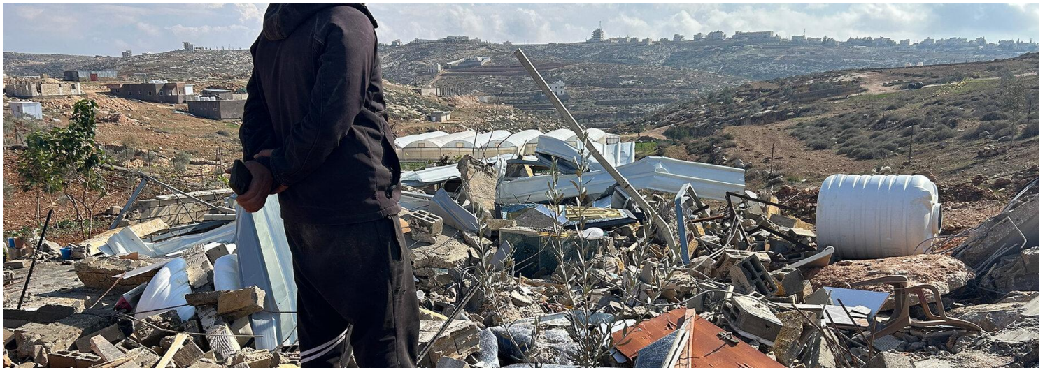
Tha'er Harb looking over what is left of his property after Israeli authorities demolished his home and five other structures in Khallet Al Farra area of As Samu' for lacking Israeli-issued building permits in Area C of the southern West Bank. Photo by OCHA, 10 December 2025.
