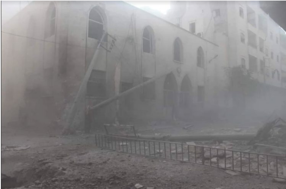
Damage caused by Syrian regime's air attack on Obada Bin al Samet Mosque in Jisr al Shoghour city, Idlib – November 7, 2019.
