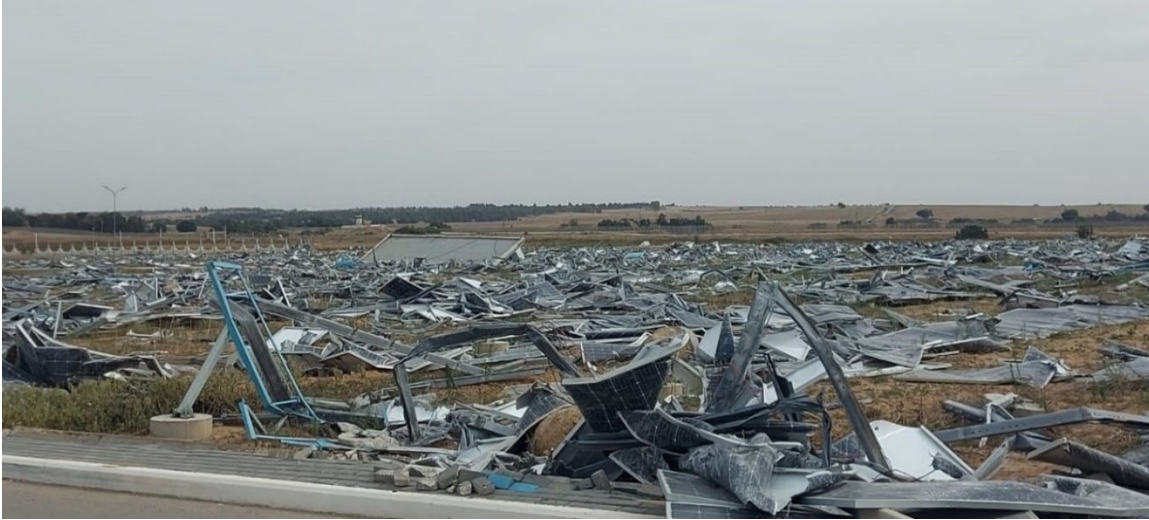
Photograph shared by a Gaza Coastal Municipal Water Utility employee with Human Rights Watch on January 16, 2024 shows the solar panel field powering the Central Gaza wastewater treatment plant completely destroyed. © Private
