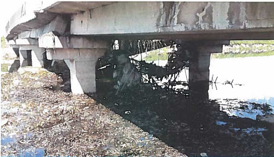
The destruction of al Twaina Bridge in Hama suburbs following the bombing by Hay'at Tahrir al Sham – April 17, 2019
