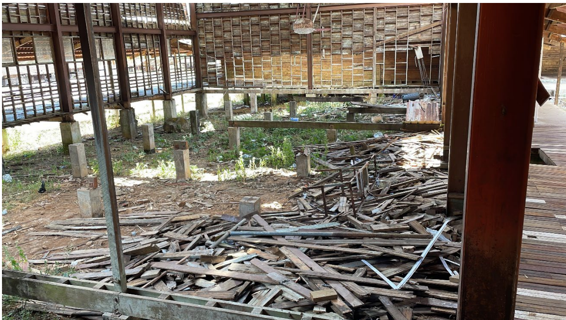
Debris from the collapsed structure of the migrant reception station of Planes de Gualaca, Panama, litter the ground. In 2023, large areas of the place were inaccessible, marked off by yellow hazard tape. The entire center was still closed as of March 2024. © 2023 Human Rights Watch
