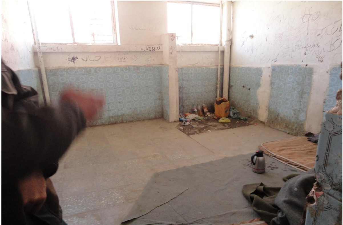
This picture shows that the situation was too bad
