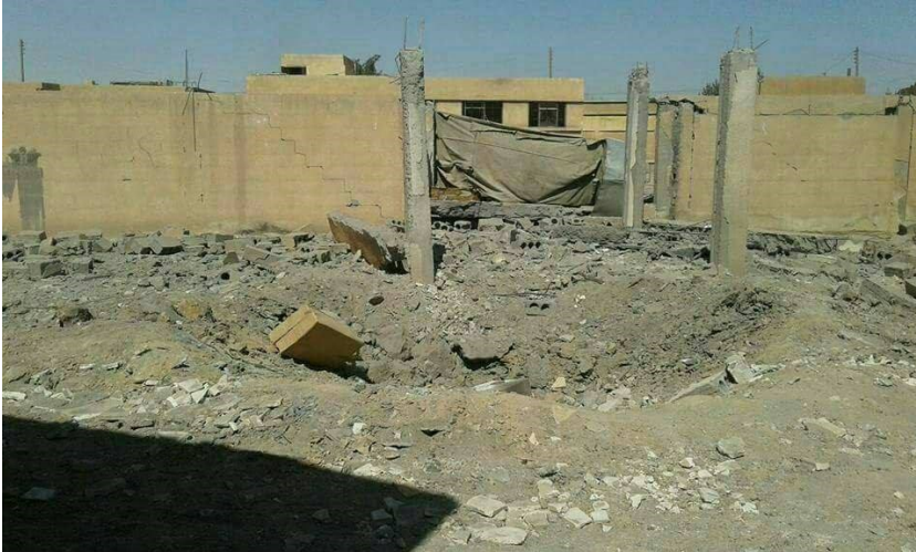
Wall collapsed because of strong wind
