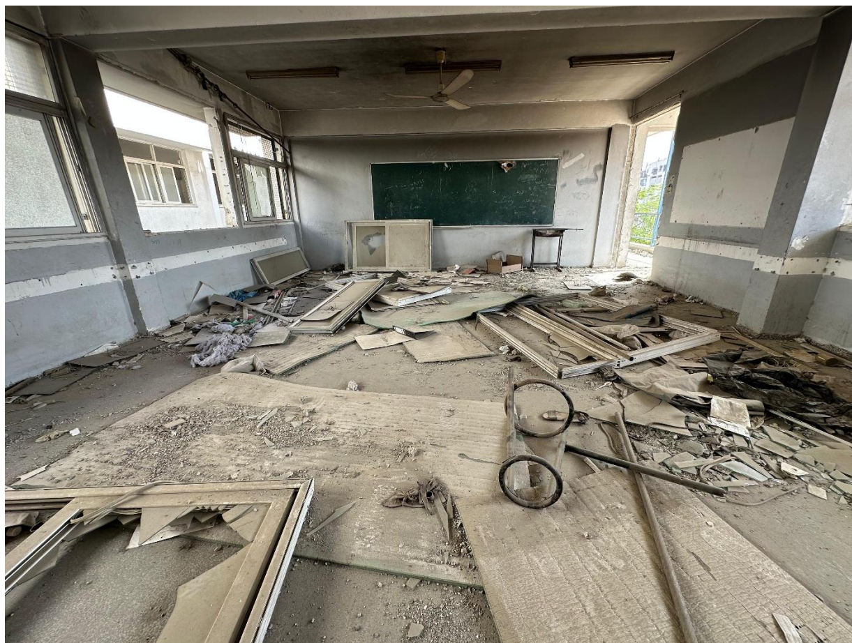
Destroyed classroom of an UNRWA school in Gaza, where students have lost access to safe learning spaces. Children in Gaza, like all children, have the right to education. Instead, they are out of school for a third year due to the war. © 2025 UNRWA photo.
